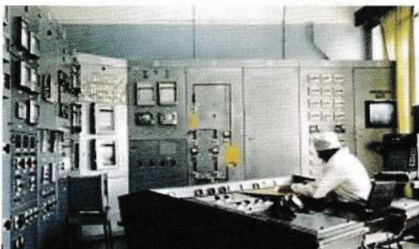
RBT-10 control room
