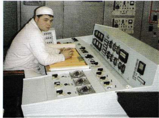
RBT-6 control room
