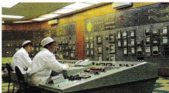
BOR-60 control room
