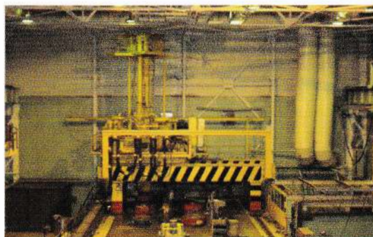
BOR-60 central room. Refueling machine
