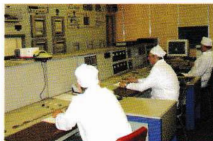
V-1000 control panel
