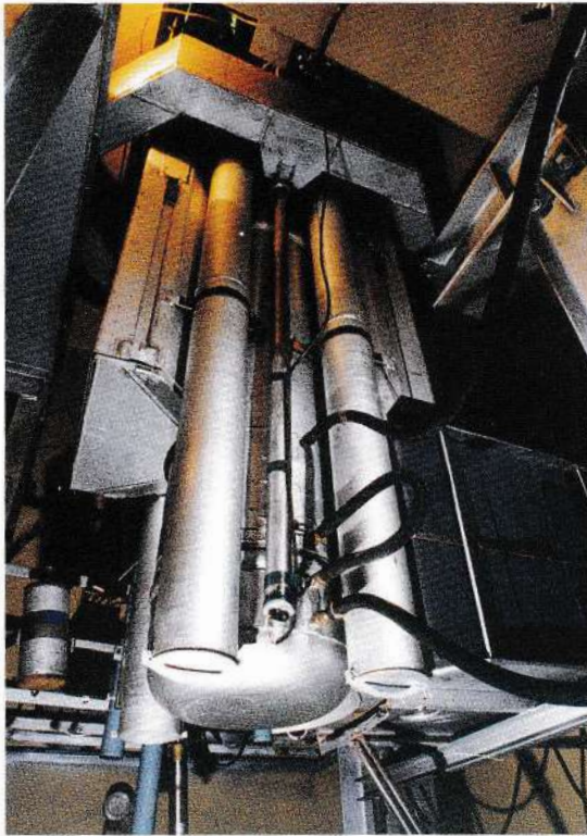
Central hall of the Gidra reactor
