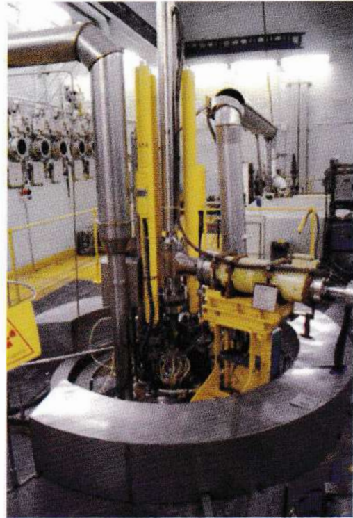
Top view of the Gamma reactor
