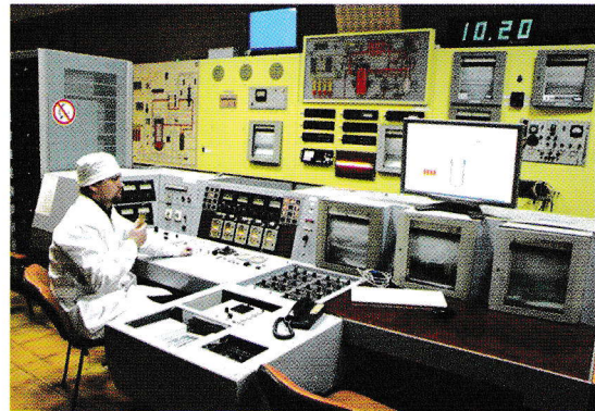
ST-1125 control room
