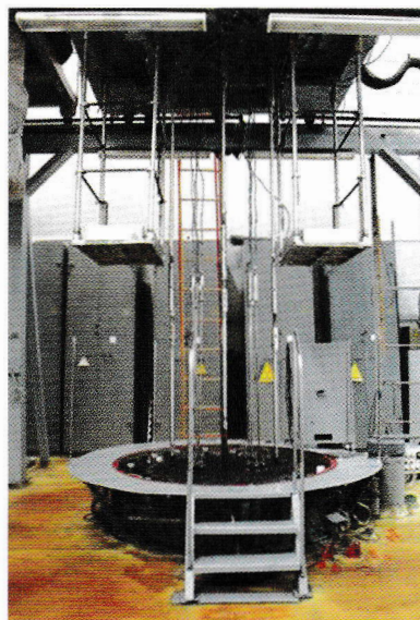
Overall view of the ST-659 facility
