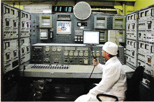
ST-659 control room
