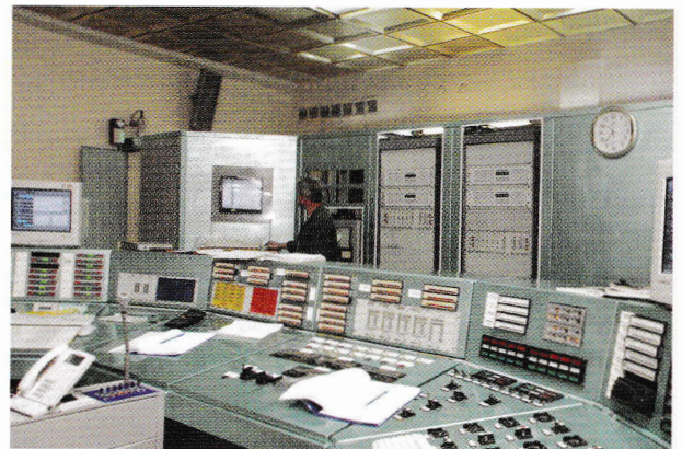
Upgraded IRT-T control room
