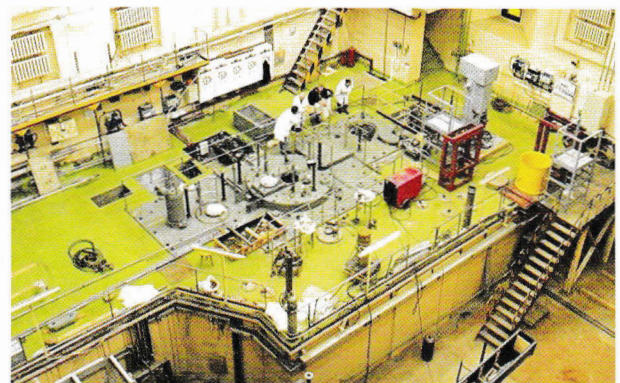
IRV-M2 reactor hall
