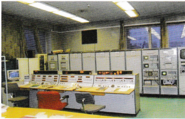
BARS-4 reactor control room
