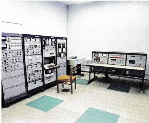
GIR-2 control room
