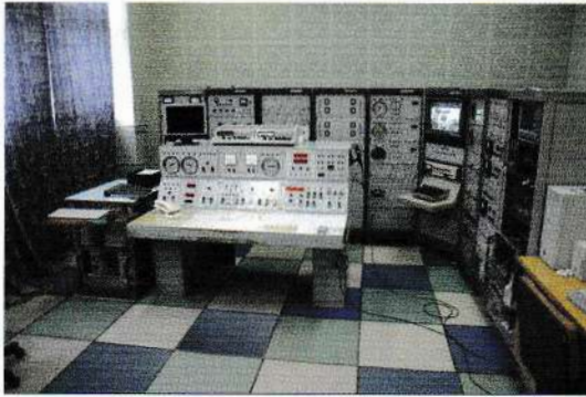
BR-1M control room
