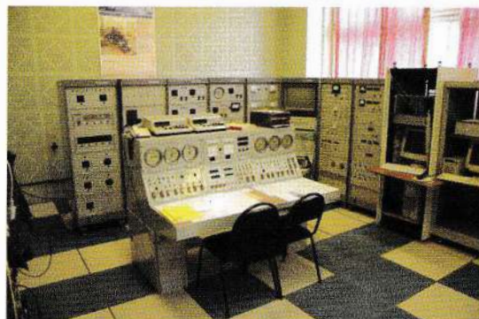
BR-K1 control room
