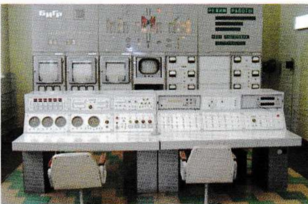
BIGR control room
