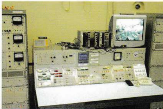
FKBN-2M control room
