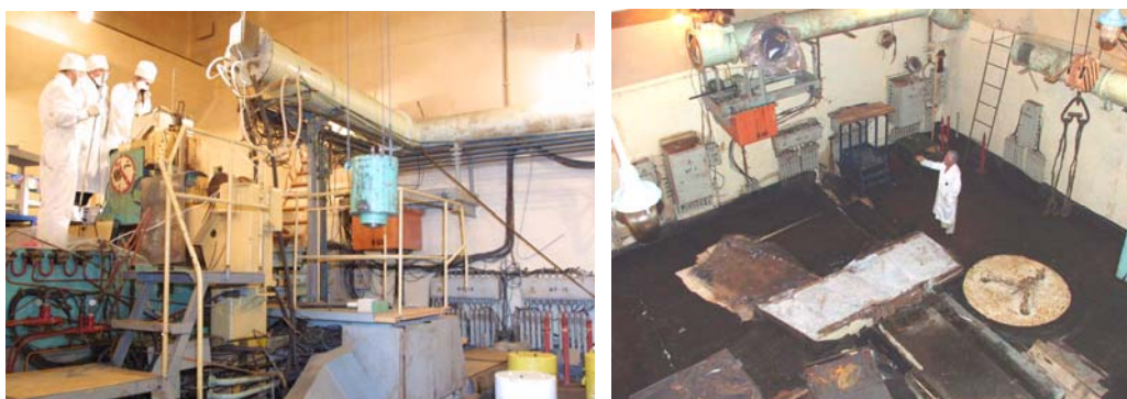
Fig. 1. The IBR-30 reactor hall in the process of fuel assembly unloading and after the preparation to the repair.
