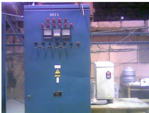
Fig.15. Power electric drives EKT2 (left) and EKT4 (right).
